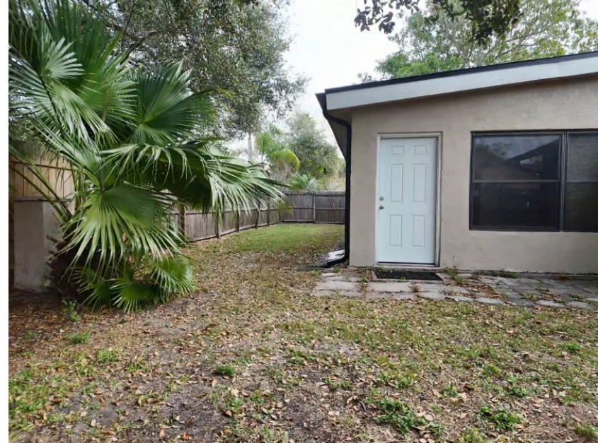
Unprotected Solid Entry Door
